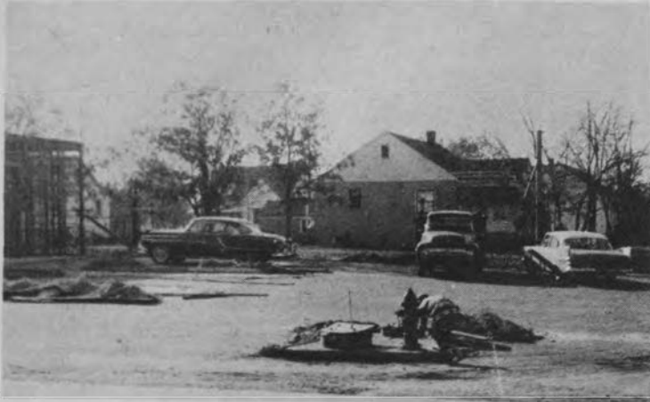
WORK AS USUAL: Workman putting finishing touches on station despite Madison Township Committee order revoking Building Permit. Township will seek a stop order this week.
